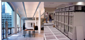
Energy Saving Smart Grid
