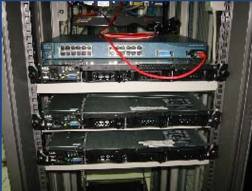
Front of Node Routers, Switches, (serial console), hosts
