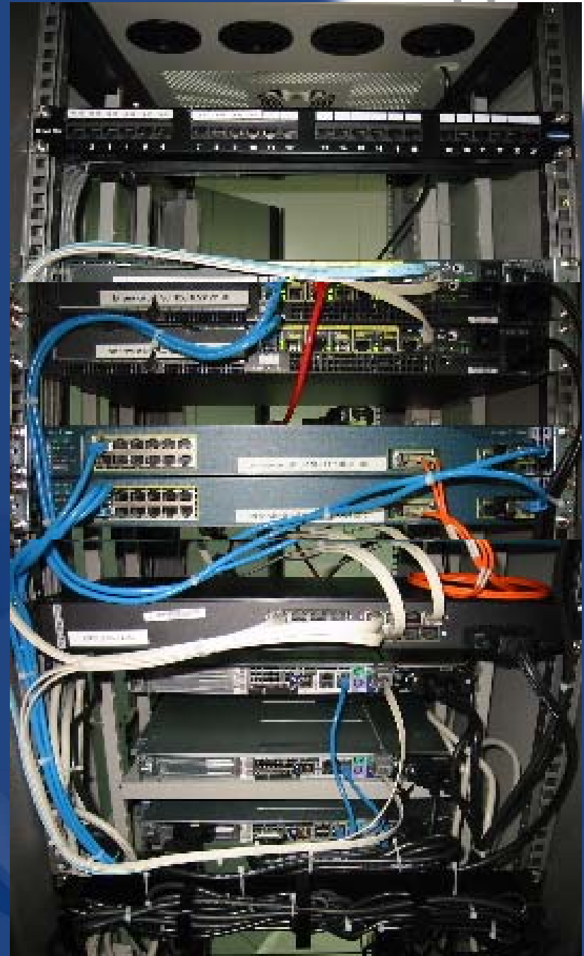
Back of Node Local media conversion (ZX to SX), hosts
